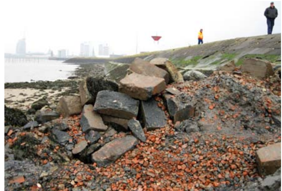
Havarieschaden am Seedeich
